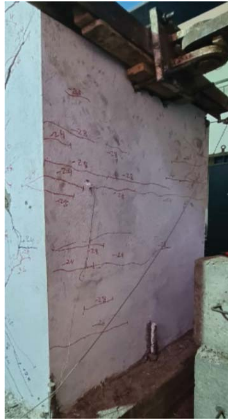
Fig. 20 Failure crack pattern S-02 (right)
